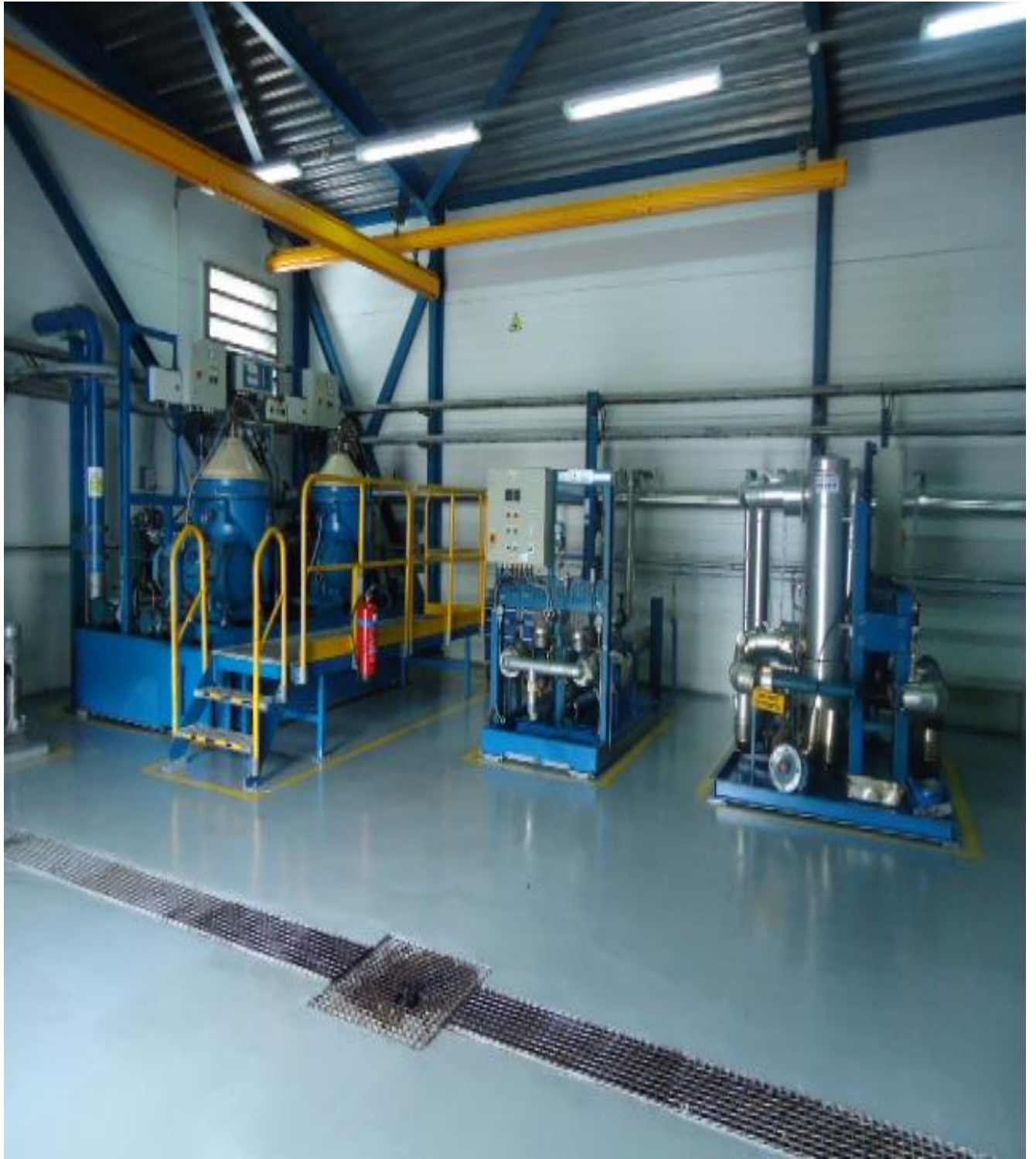
Figure 7 - Fuel Oil Purifiers
