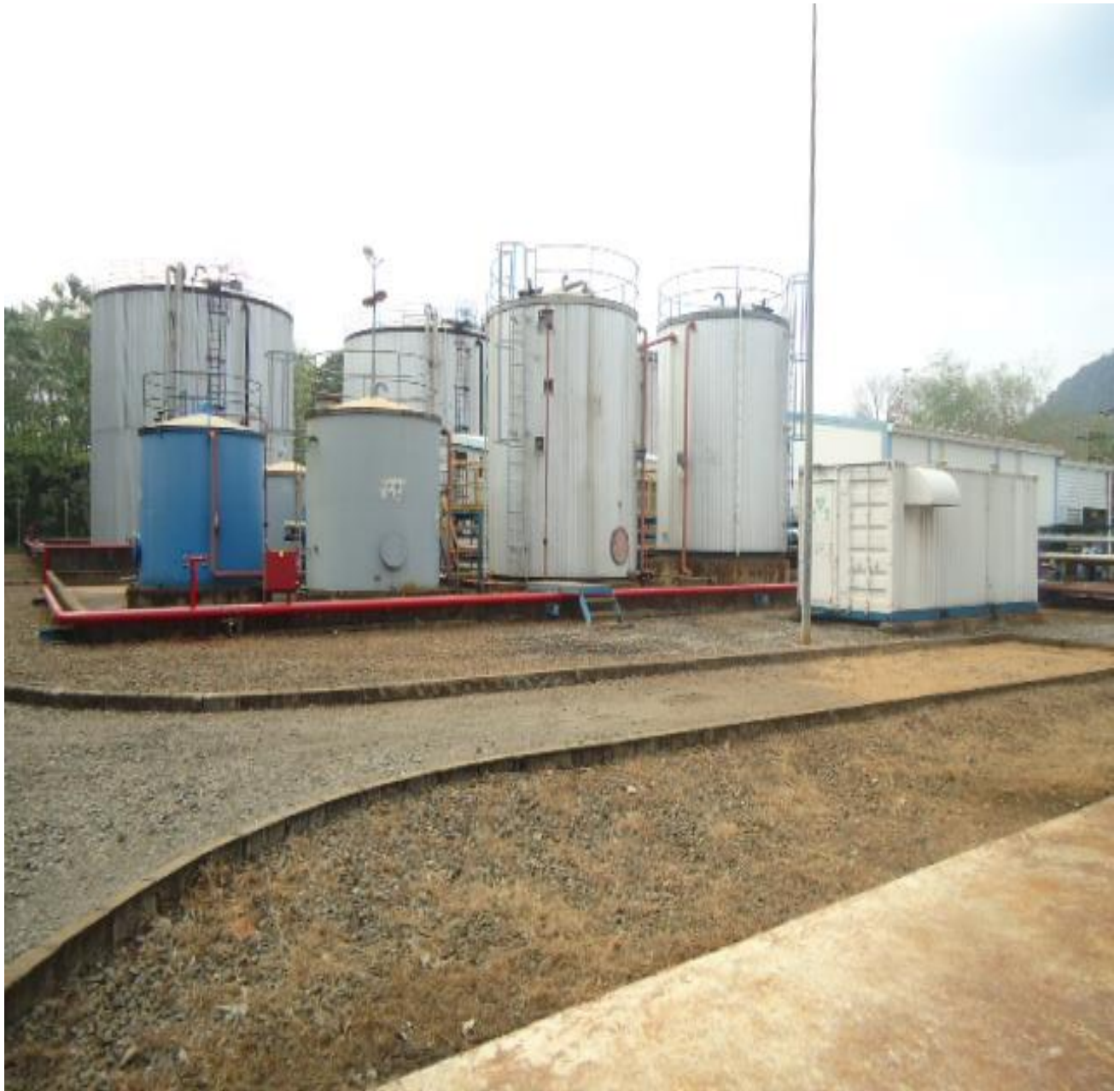
Figure 10 - Oil Storage Tank Yard
