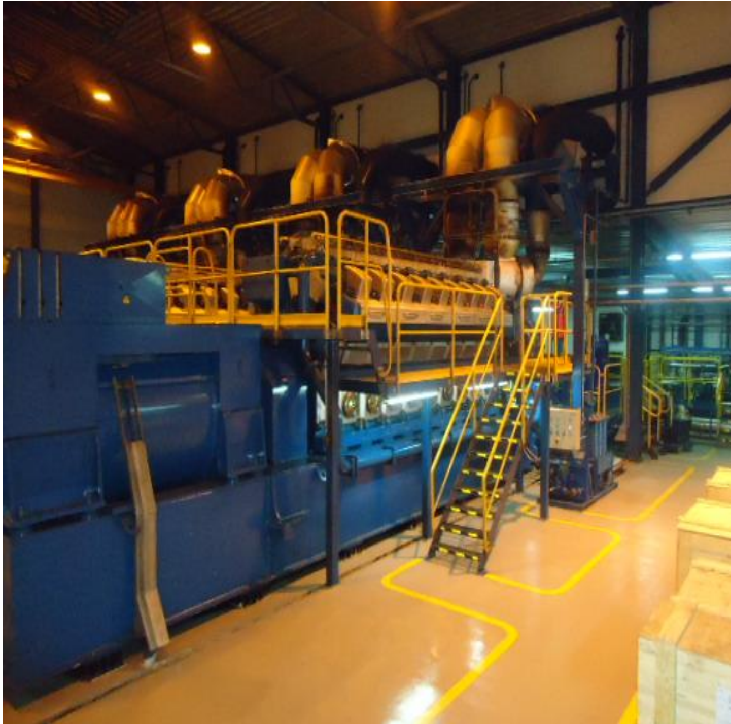
Figure 5 - DG Set Side View
