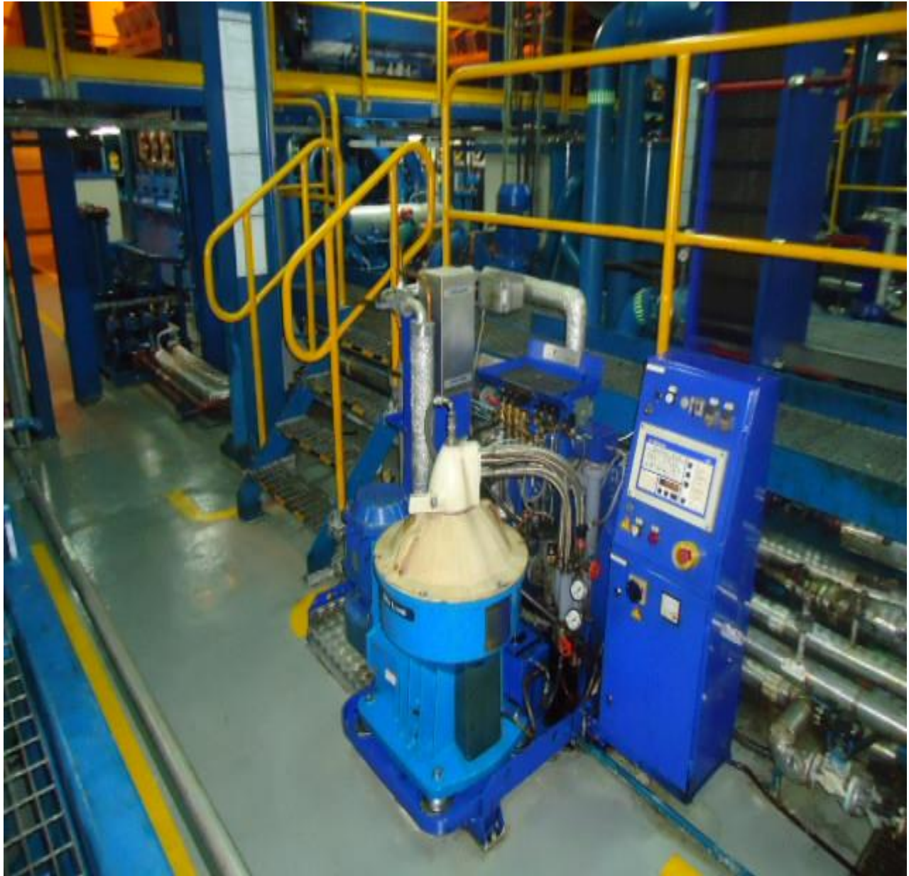
Figure 6 - Lubrication Oil Purifier
