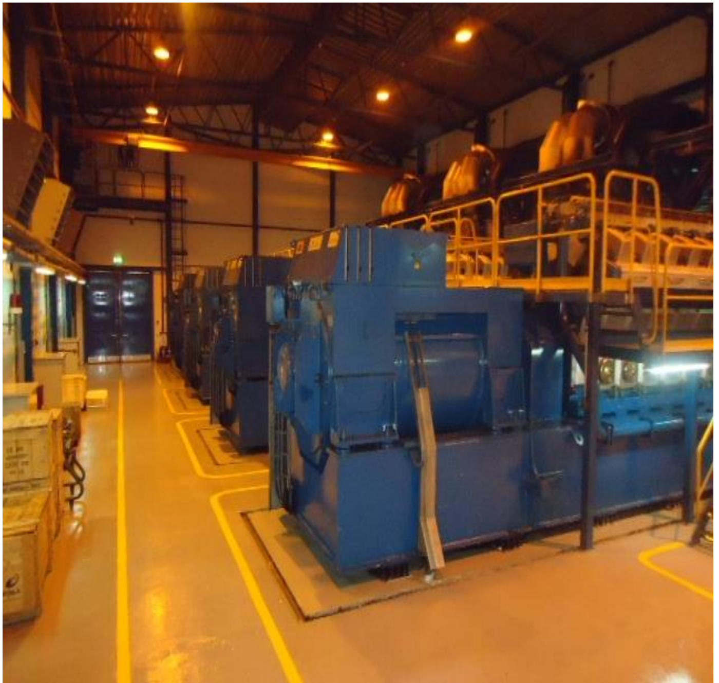
Figure 4 - Engine Room Generator Side View
