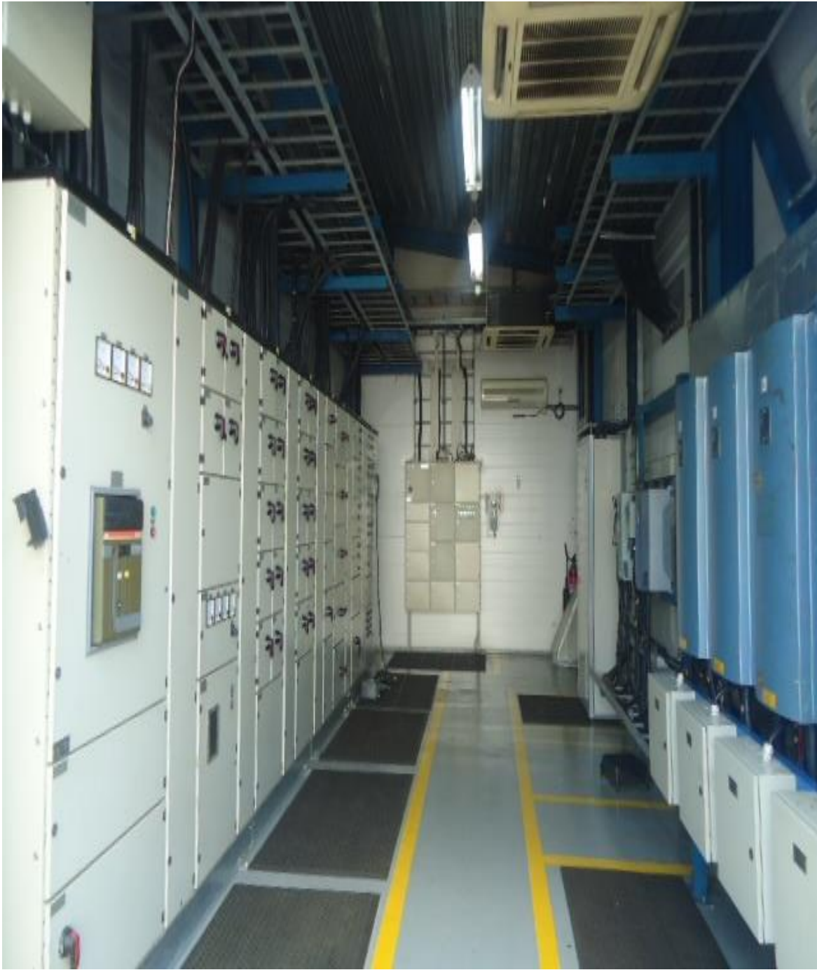
Figure 13 - LV Room Panels
