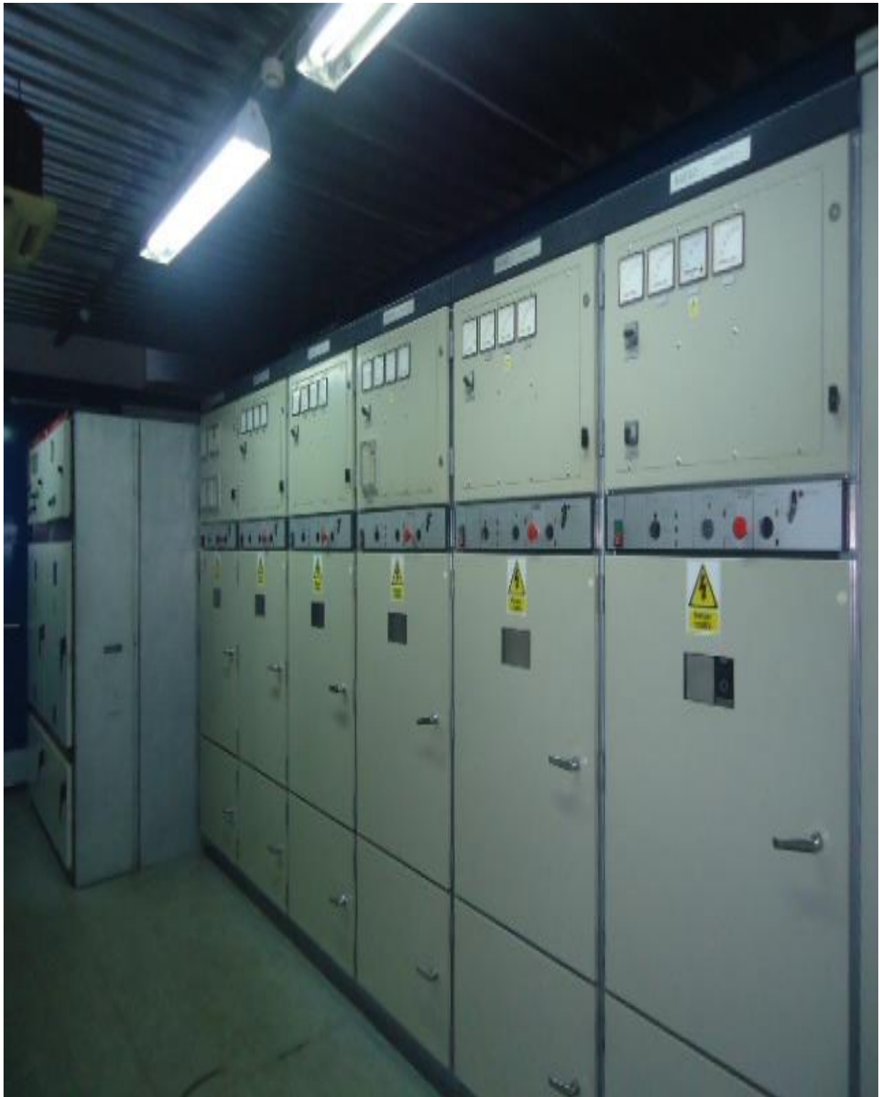
Figure 14 - MV Room Panels
