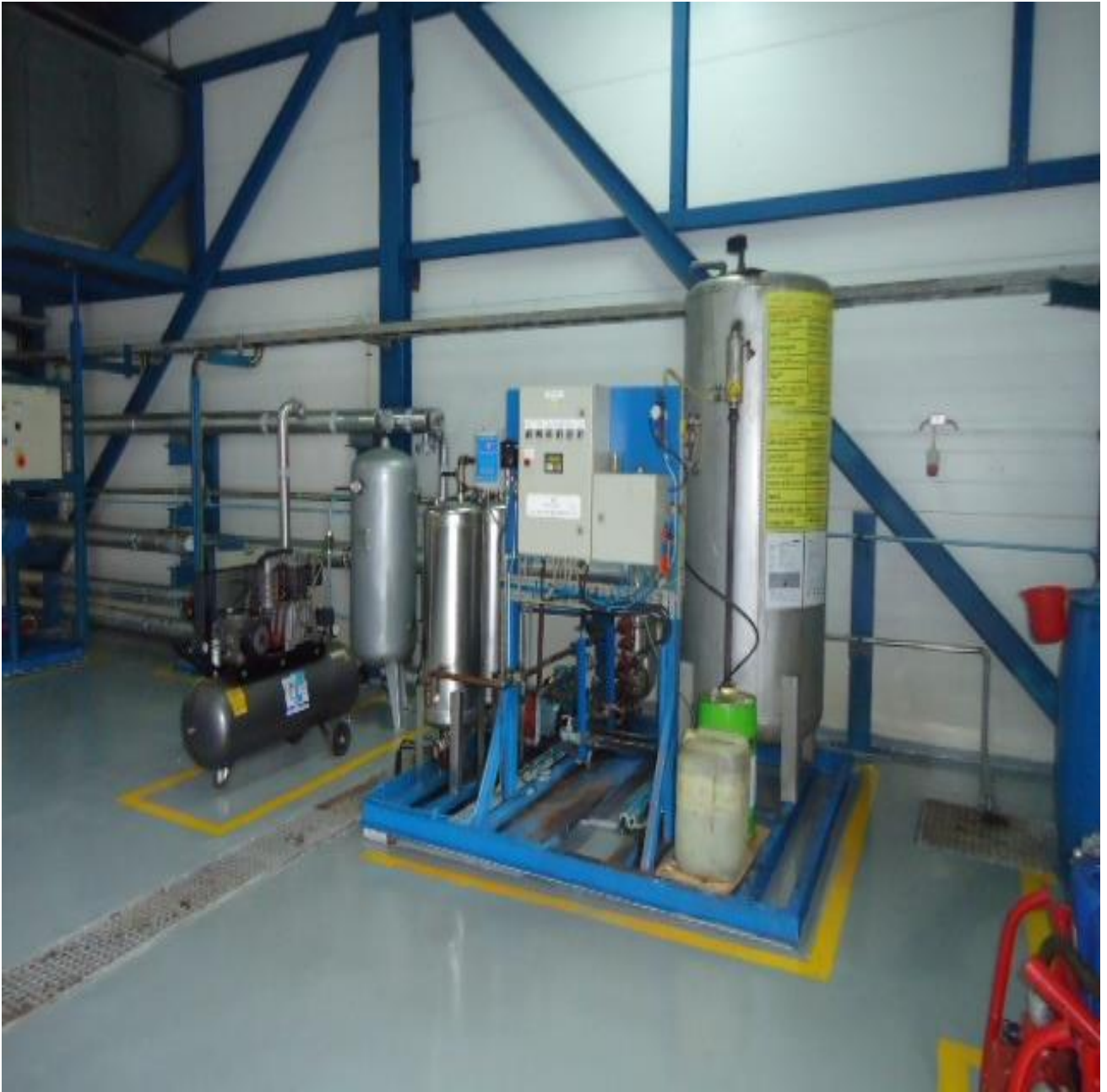
Figure 8 - Waste Water Purifier
