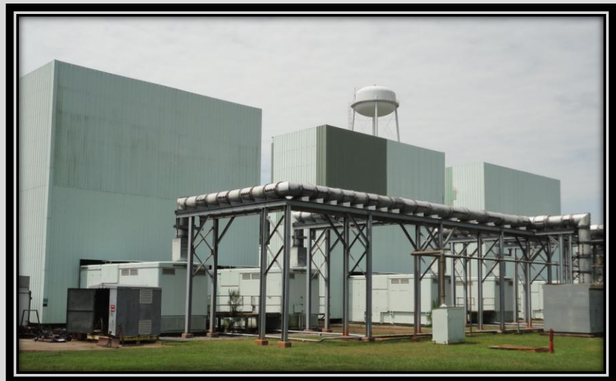
Six (6) GE Gas Turbine Generators – AFT View
