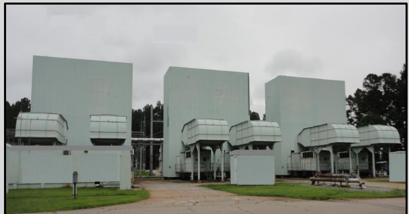
Six (6) GE Gas Turbine Generators – Forward View
