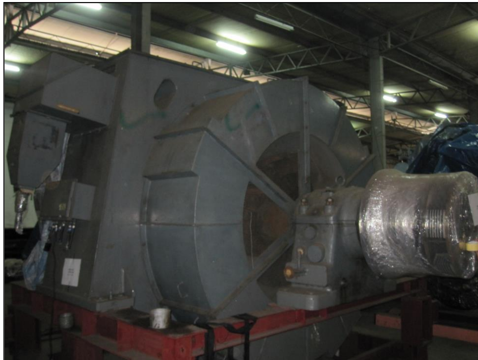
Photo No. 2 of Alternator
