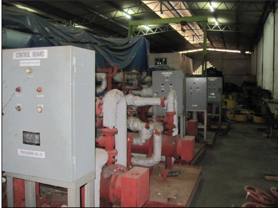
Photo of Control Board Panels
