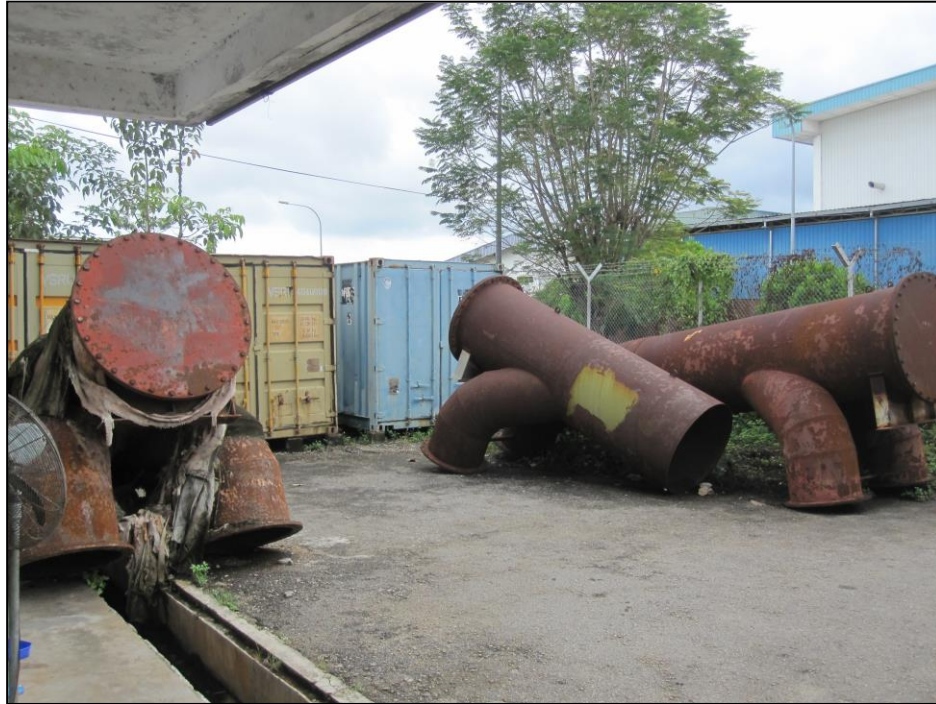
Photo of Exhaust Pipings
