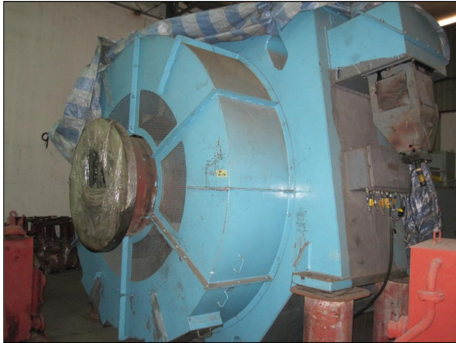
Photo No. 1 of Alternator
