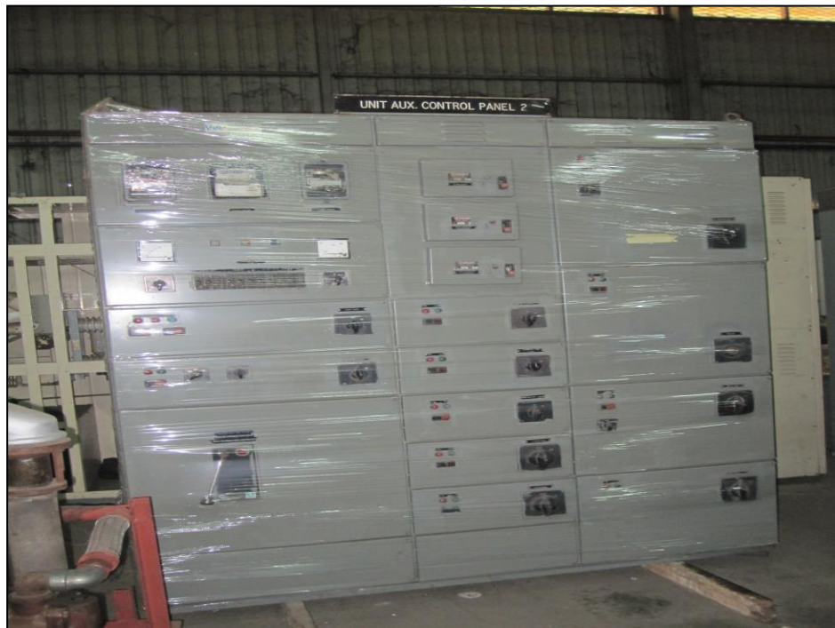
Photo of AUX Control Panel
