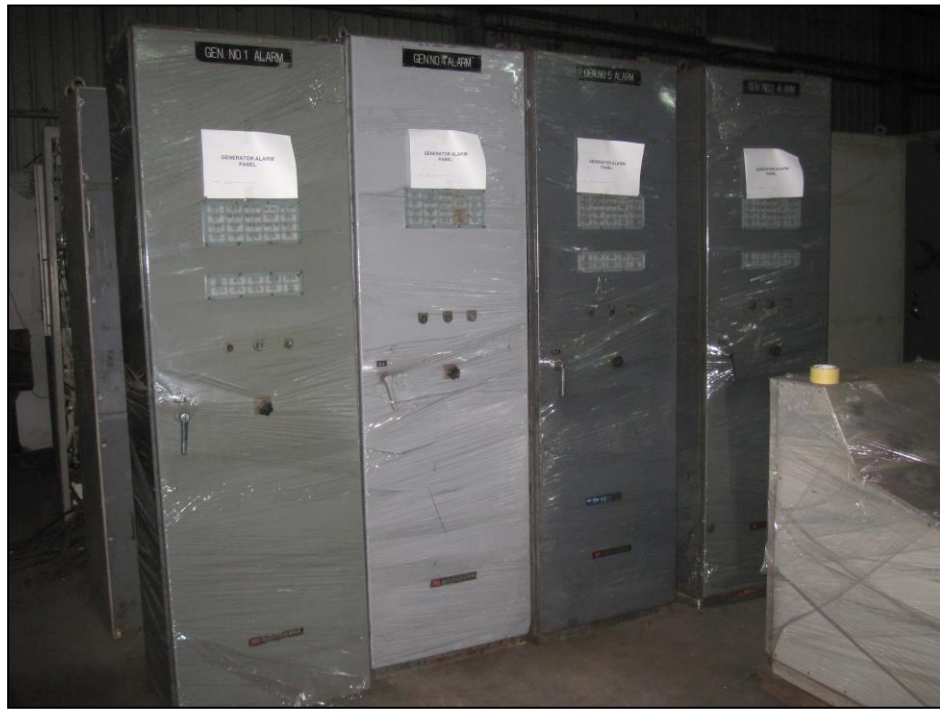
Photo of Generator Alarm Panels
