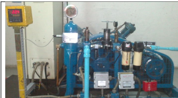
17) Starting air compressor
