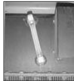
RADIATOR FLUID LEVEL GAUGE
