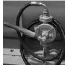
WASTE OIL/SUMP PUMP
