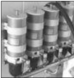
PRIMARY FUEL FILTERS (RACOR)
