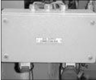
AUX SUPPLY CONNECTION BOX
