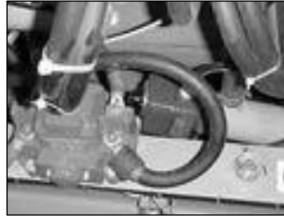
BATTERY ISOLATOR BLOCK WATER HEATER
